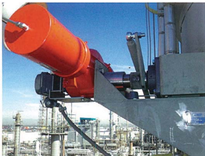
Actuator and controls upgrade to provide better precision to stack damper movements
